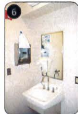
Bathing room handwash sink
