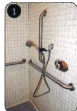
Shower room fixtures
