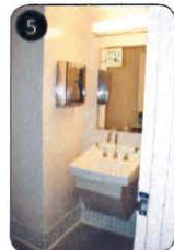
Shower room handwash sink
