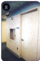
Fire extinguisher cabinet
