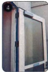
Terrace door hardware
